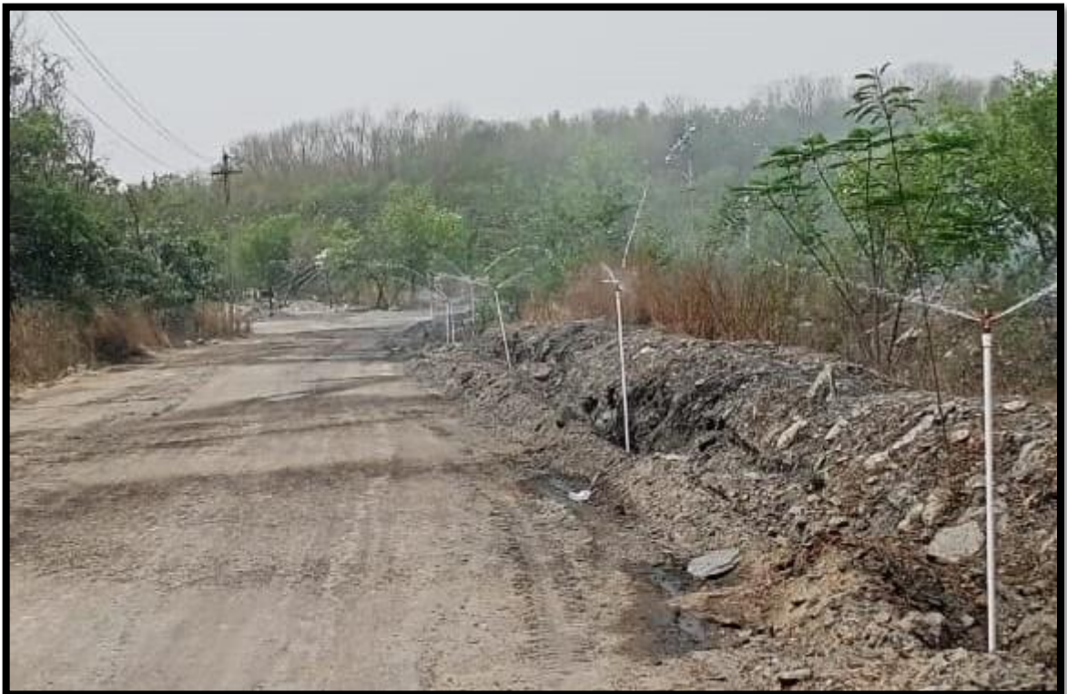
Fig 05 i- Fixed Type Water Sprinkler along Haul Road
