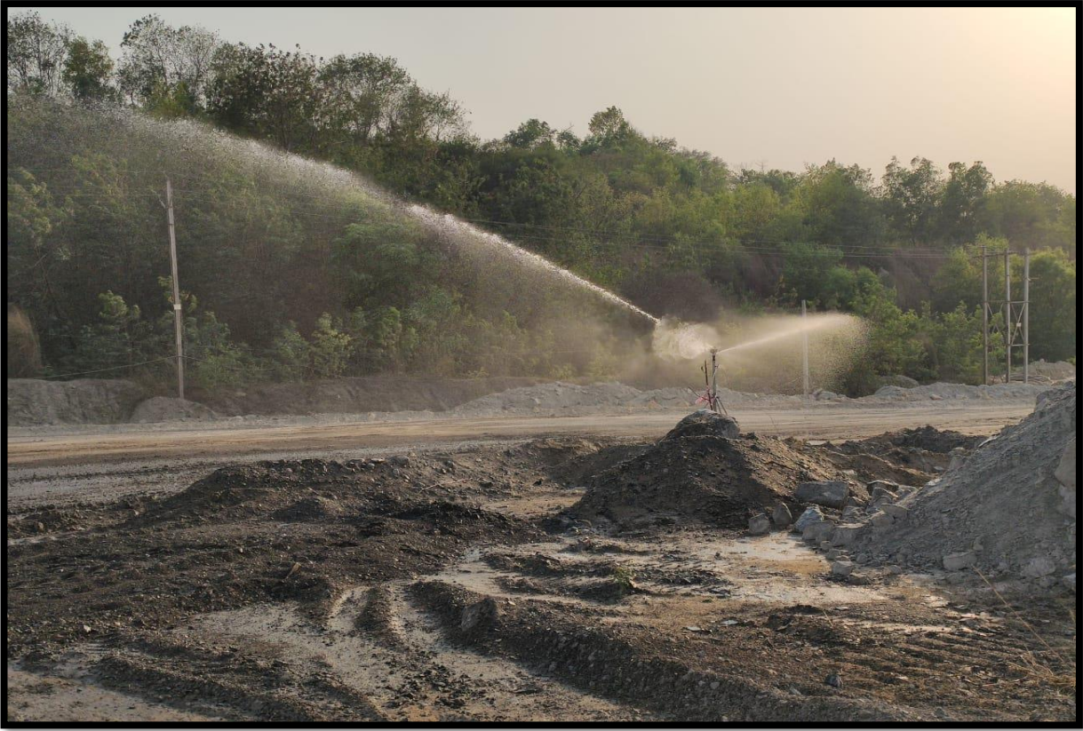
Fig 05 ii- Fixed Type Water Sprinkler along Haul Road
